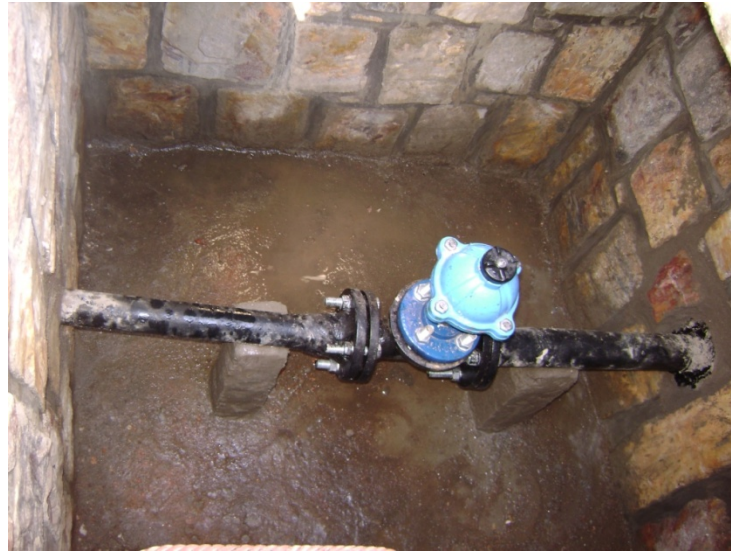
Figure 17: Picture of an air release valve
