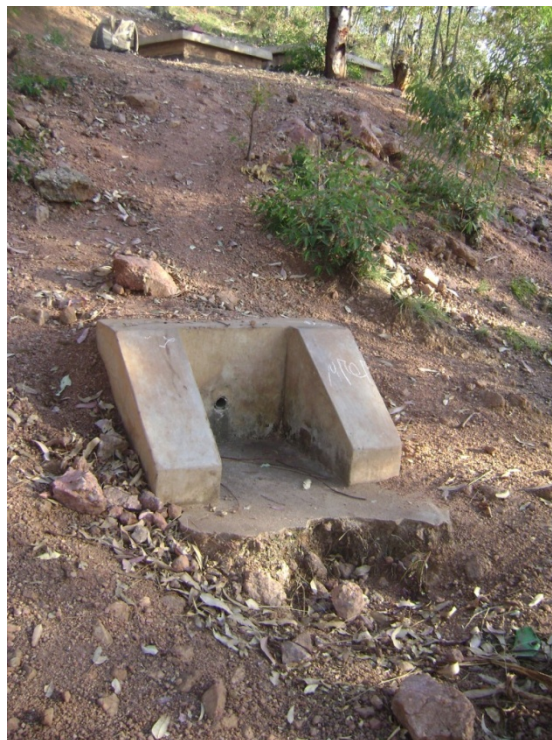
Figure 18: Soak away / tail end of a washout
