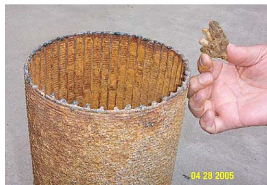
Incrustation on the well screen
