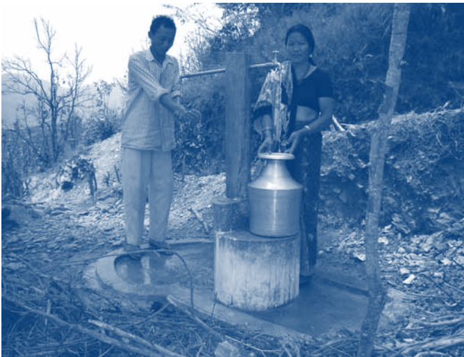
Figure 3.12. Two off-takes at a standpipe in Nepal (photo: Bimala Colavito)
