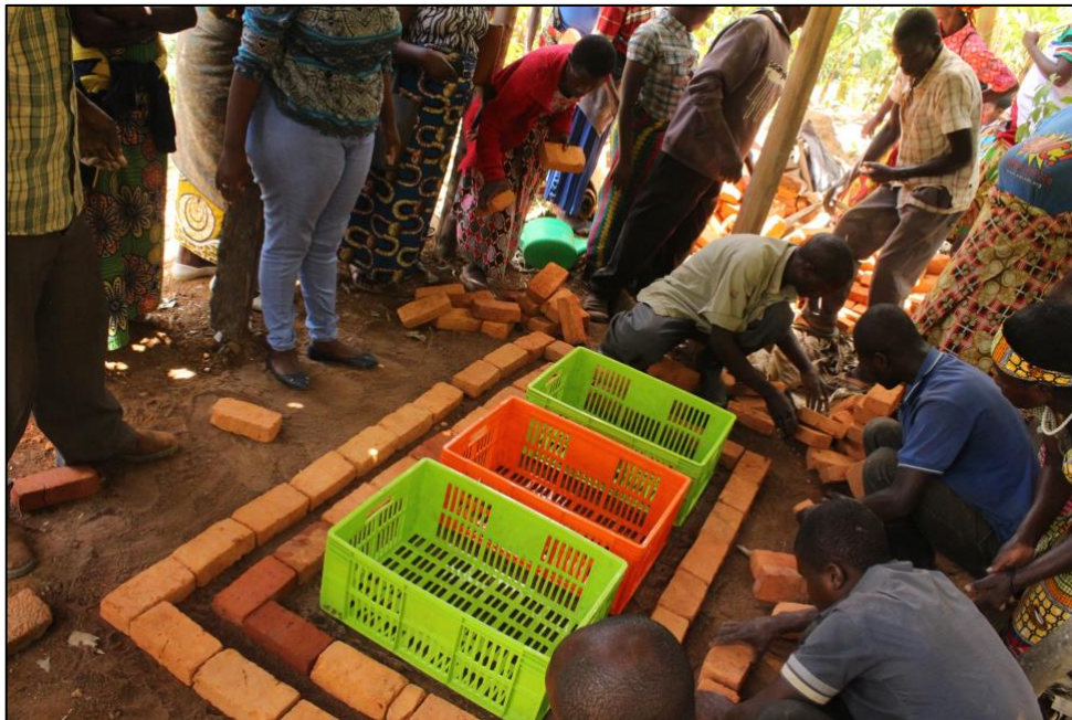
Figure 11. Construction of a brick Zero Energy Cooling Chamber by cooperative members in Gakenke, Rwanda.
