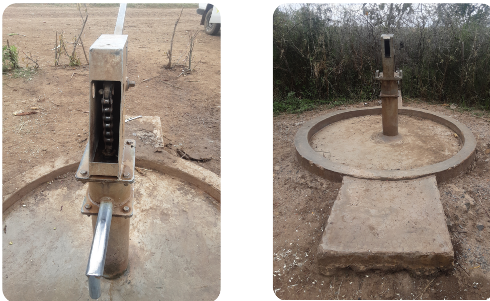
Figure 3. A pump in Karamoja missing its inspection cover and bolts (L) and a vandalized pump with the handle taken for use in plowing (R).
